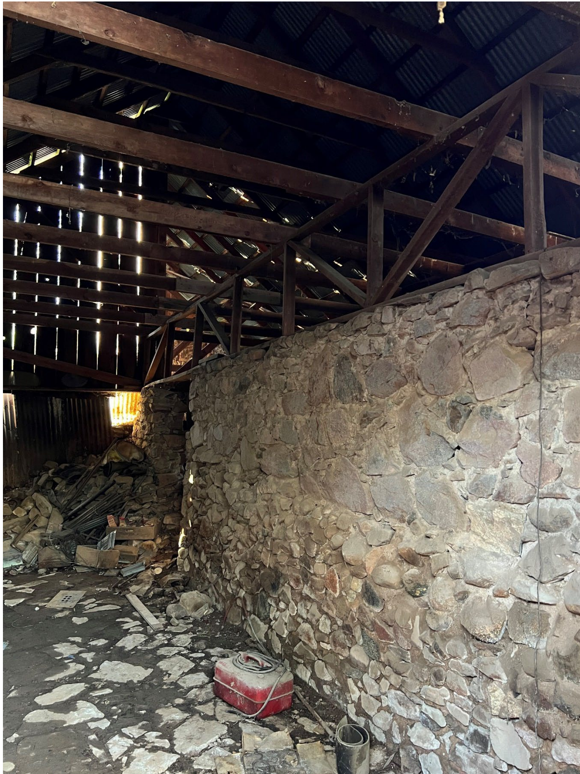
Photo #18: View of the trussed roof in the front portion of the Winery building.
