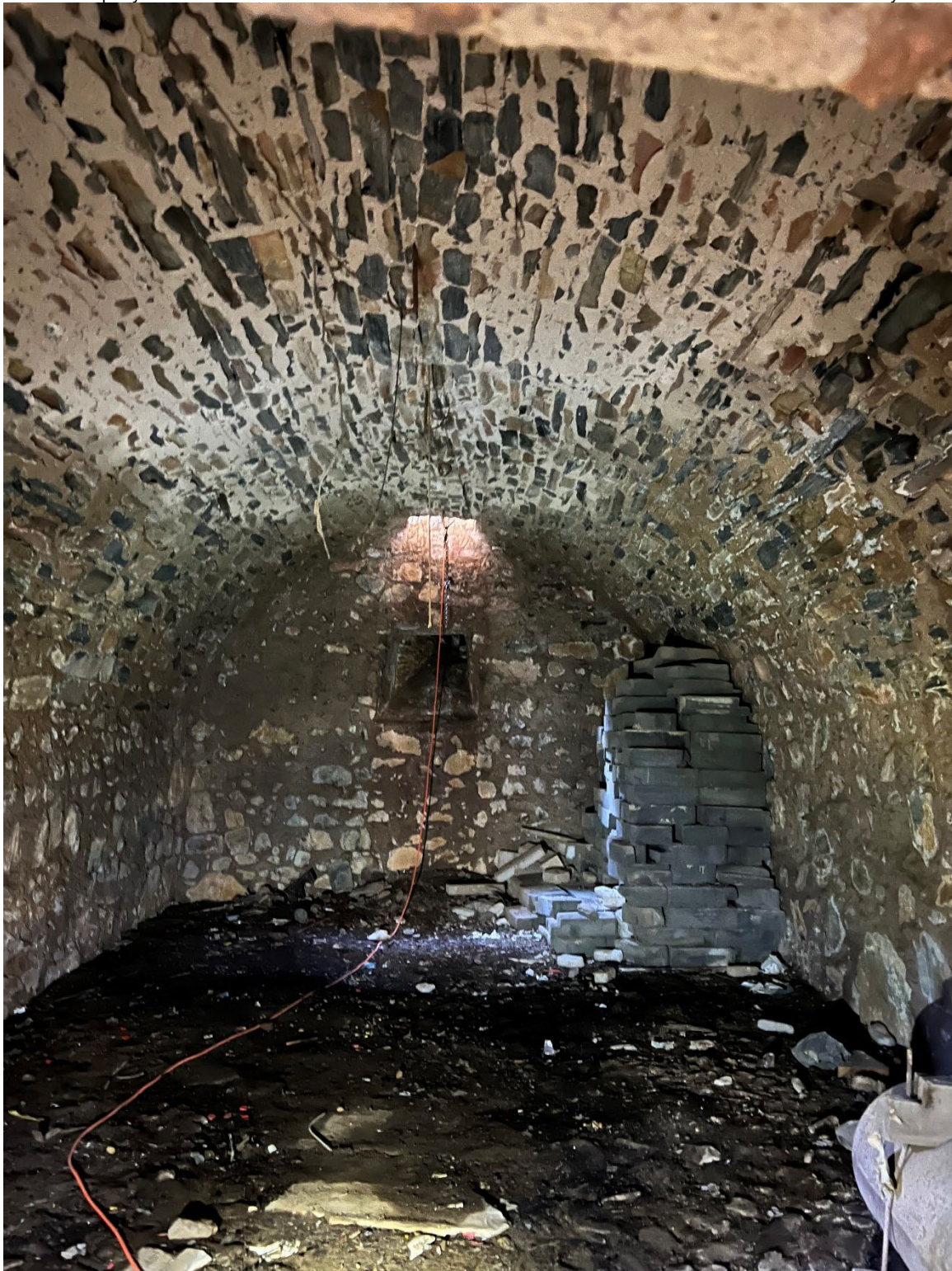
Photo #17: Interior view of the arched underground storage portion of the Winery.
