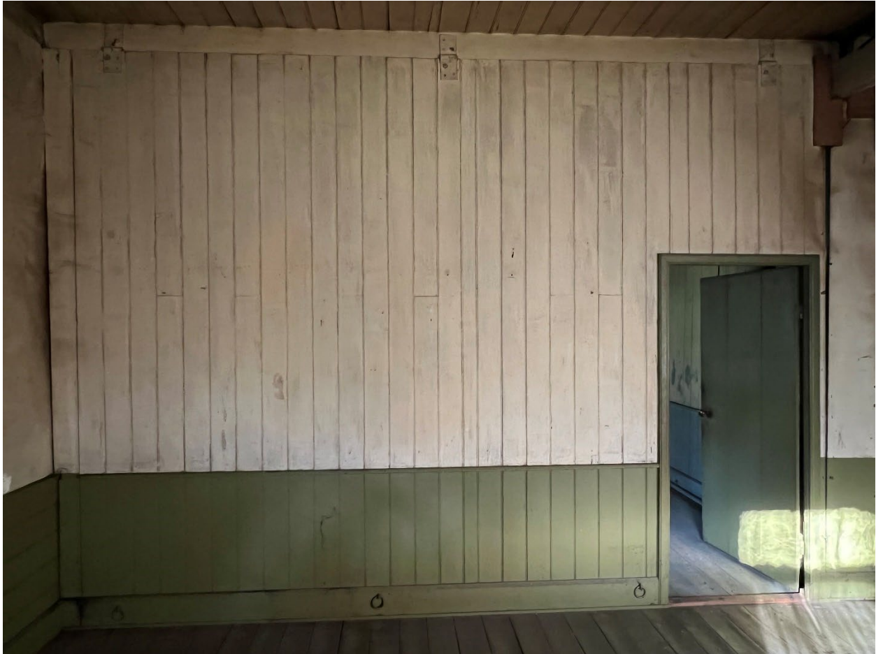
Photo #10: View of an interior partition wall. Note hinges at the top of the wall, rings at the base.
